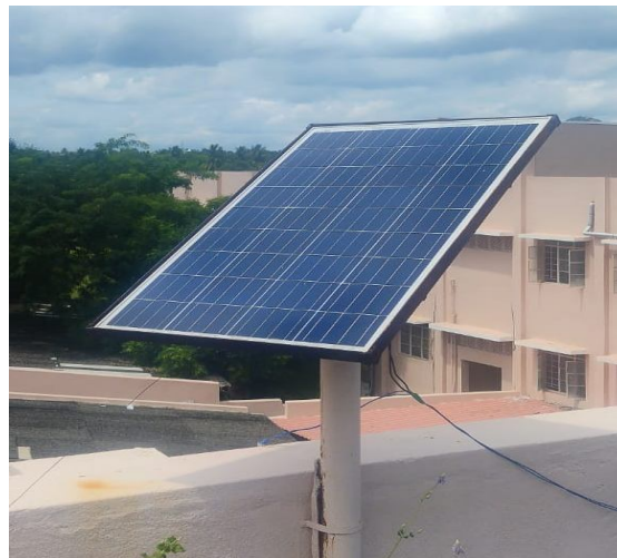
Fig 7- 100 W, 12 V solar panel
